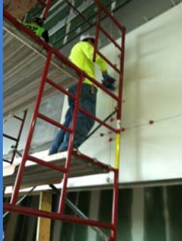
Adjusting Levelers For Perfect Alignment After Placing Back-Buttered Panel onto Wall Troweled With Thinset Mortar
