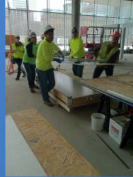
Moving Panels From Crate To Prep Table (Using Aluminum Frame w/Suction Cups)
